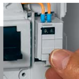
Auxiliaries are installed in dedicated locations under the front panel.
